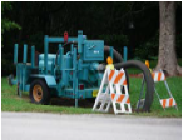
Portable stormwater pump placed prior to a predicted storm.
