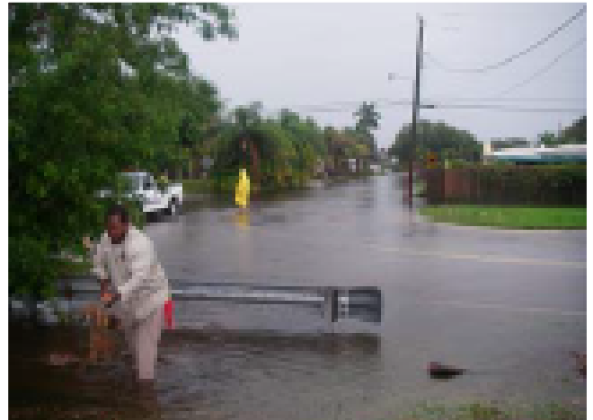
Utility field worker clearing a clogged storm drain on a flooded street.
